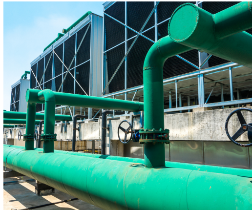
Water Treatment Facility
